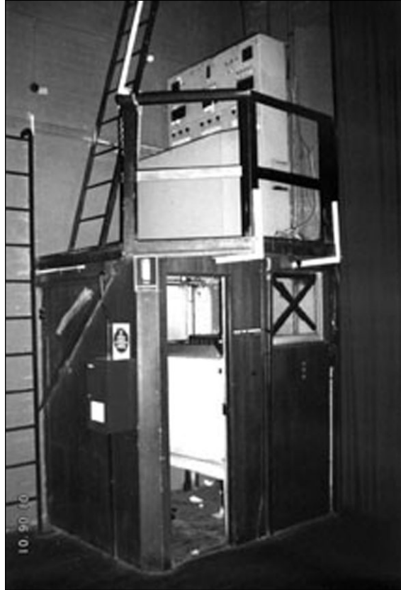
Figure 69. Stage control box at front of Campbell Street side of stage.
