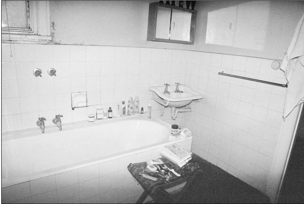
Figure 61. Substandard bathroom in caretaker's flat.
