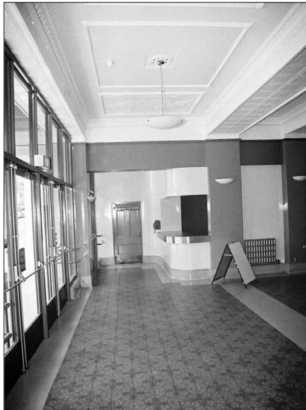
Figure 55. View of foyer showing counter. Note the missing panel of pressed metal in the ceiling around the light.
